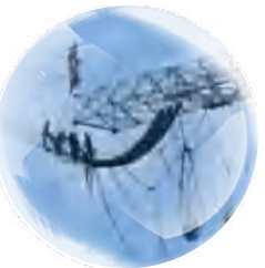
South Hami-Zhengzhou ± 800kV EHV DC Power Transmission Line Project
