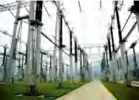
Large cross-section bare conductor of JL1/G3A-1250/70 had been used in the Changji - Guquan \pm 1100kV Transmission line Project
