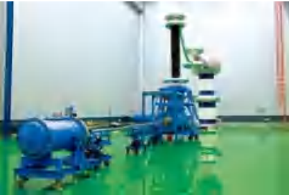
220kV Ex-work Test Equipment
