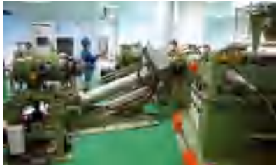
35kV Continuous Vulcanization Line From Germany
