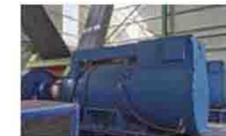
· Application of Belt Conveyor in Qingdao Steel Plant
