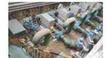
· 400kw Blast Furnace Pump of Shiheng Special Steel
