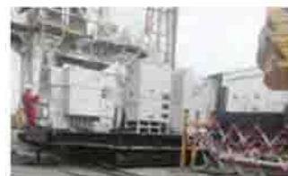
· Drilling Platform Mud Pump
