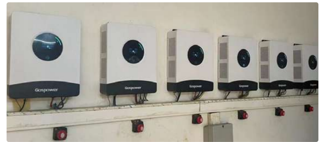
6 x Gospower 6kw Inverter Three phase system
