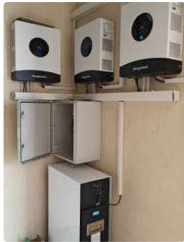
3 x Gospower 6kw Inverter 1 x Gospower 15kWh Lithium Battery
