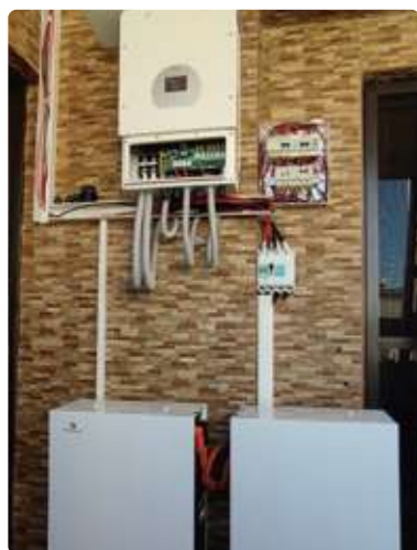
1 x 8kw Inverter 2 x Gospower 15kWh Lithium Battery
