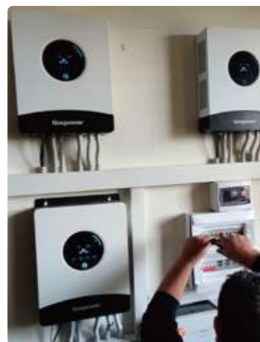
3 x Gospower 6kw Inverter 1 x 10kWh Lithium Battery
