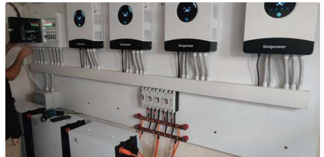
4 x Gospower 6kw inverters 3 x Gospower 15kwh lithium battery
