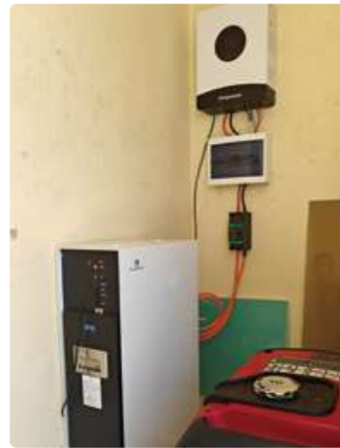
1 x Gospower 6kw Inverter 1 x Gospower 15kWh Lithium Battery
