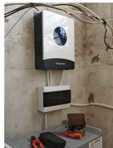
1 x Gospower 6kw Inverter 1 x 15kWh Lithium Battery
