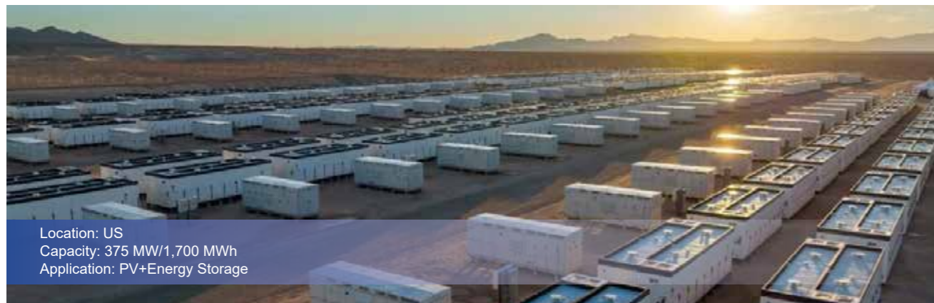
Location: US Capacity: 375 MW/1,500 MWh Application: PV+Energy Storage
