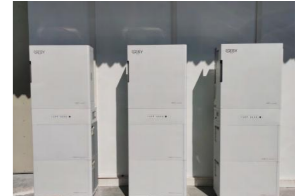
Installation in Belgium
