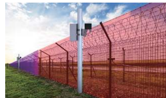
Airport Perimeter Security System
