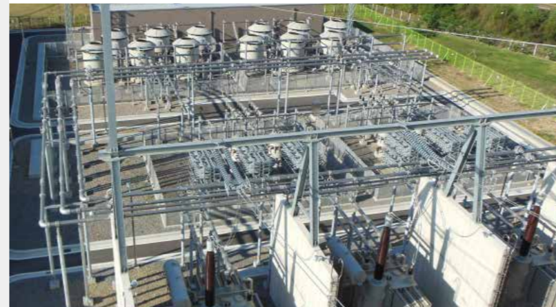
-200MVar ~ +200MVar SVC project in Korea
