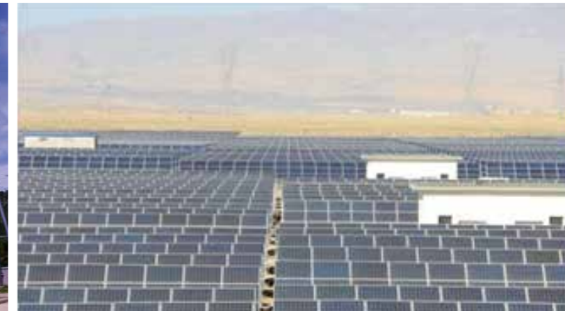
20MWp PV generation project in Qinghai
