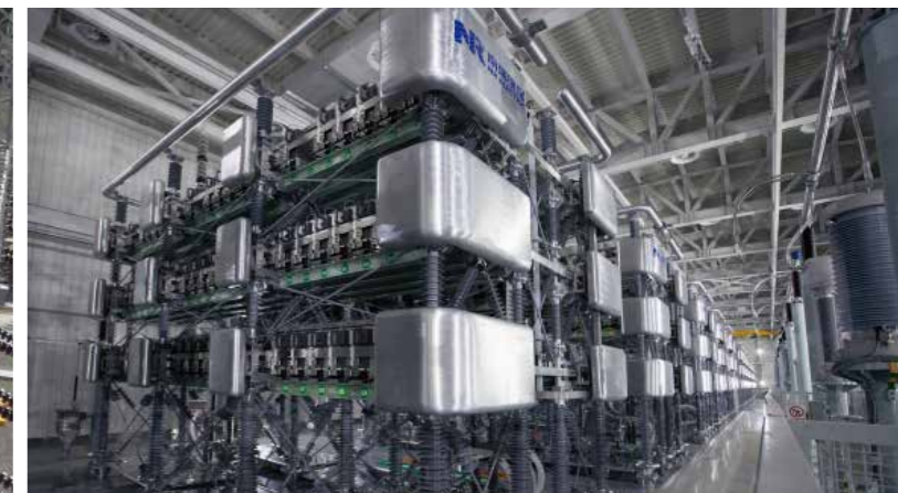
500kV 750MVA UPFC in Suzhou China
