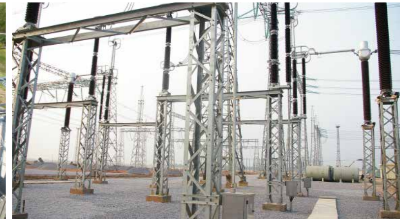
500kV substation secondary system in Vietnam
