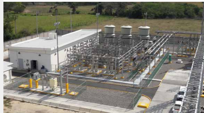
-50-150 Mvar SVC in Mexico
