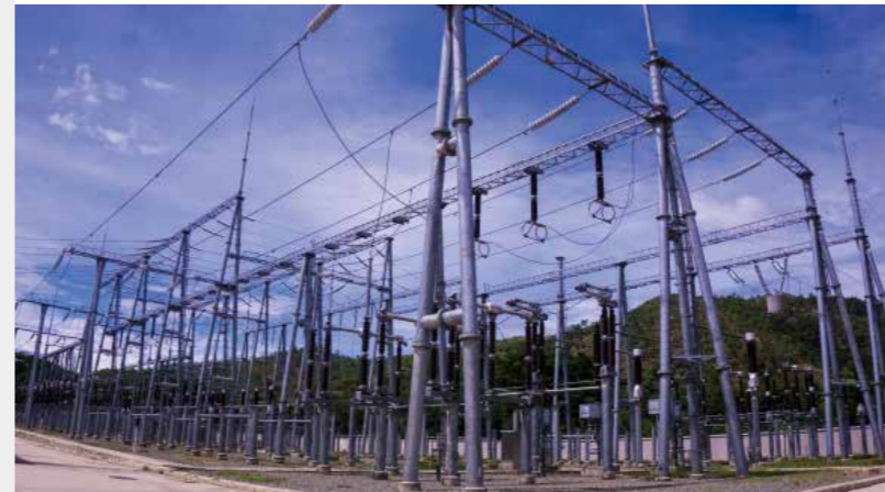
275kV Substation in Malaysia
